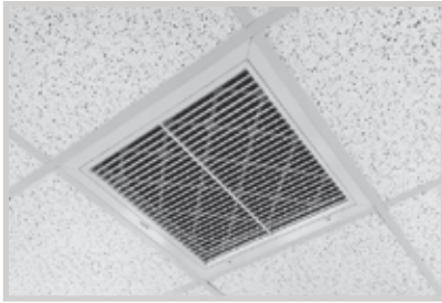
Return grill attached to filter assembly
